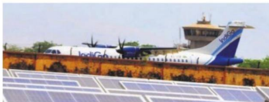
A view of the newly set up solar power plant at Tirupati airport | EXPRESS
